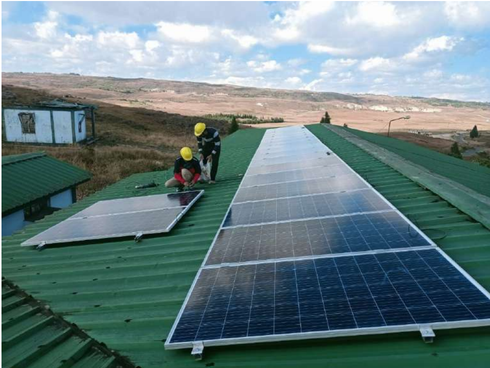
Fig- Installation of Solar Setup in Mawkynrew PHC, East Khasi Hills
